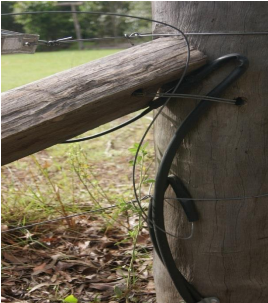
Undergate cable end detail. Note downturned ends of the poly pipe.
