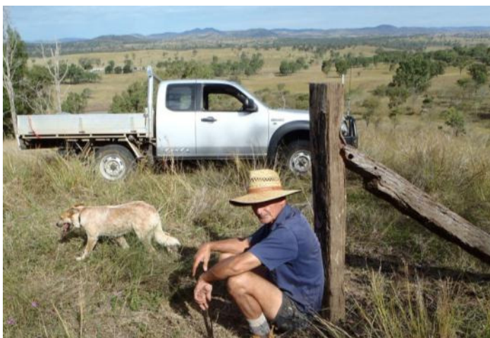
Mr Richards in the process of installing new fencing on Ewii Station
